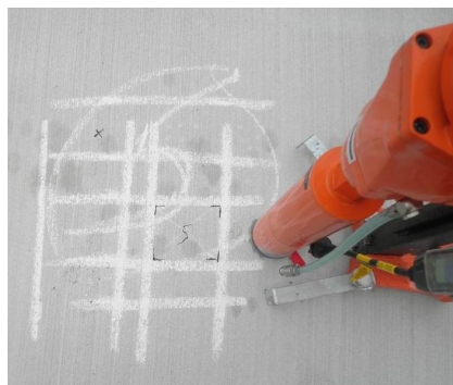
View of reinforcement location prior to core extraction for compressive strength testing.
